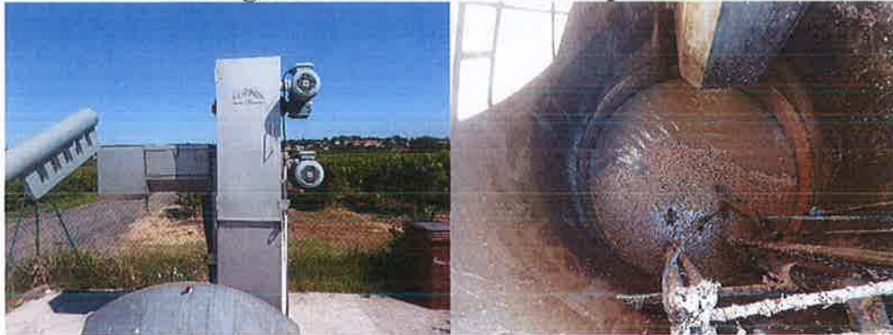
PR alimentant la station
